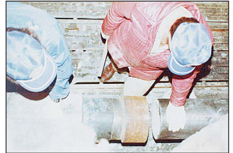
Aligning of the ends of the two pipestrings before welding the 'Tie-In' weld.
