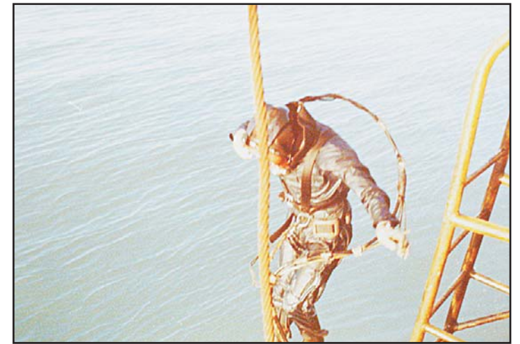
A diver controls the 'Tie-In' after the final abandoning of the pipeline.
